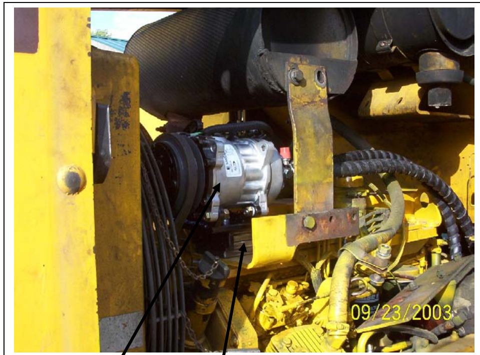
Compressor in place with 2:” 2” spacer 1/2” and 13/32” lines spacer
