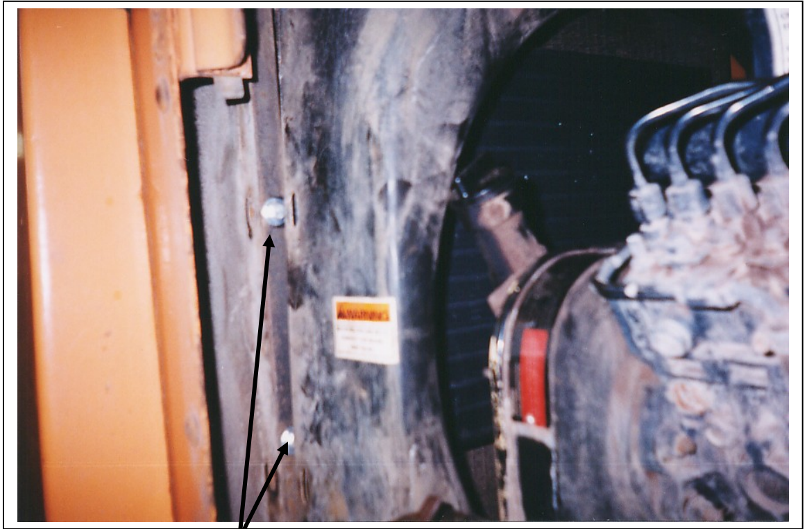
Bolts holding condenser brackets in place
